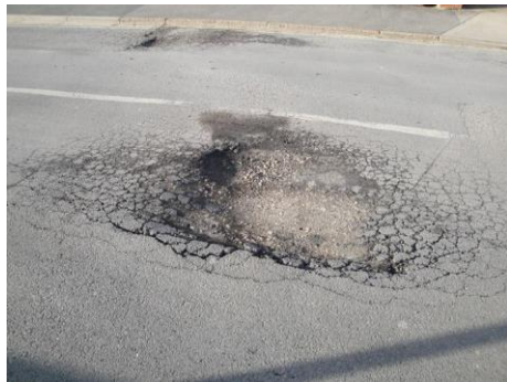
Figure 13.8: Thermal stress contributes to the formation of potholes. (credit: Editor5807, Wikimedia Commons)
