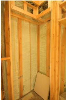
Figure 14.8: Insulation is used to limit the conduction of heat from the inside to the outside (in winters) and from the outside to the inside (in summers). (credit: Giles Douglas)
